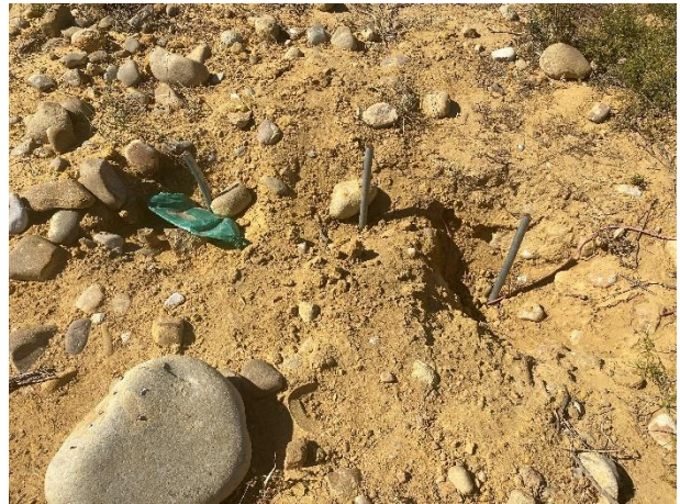
Exposed steel wires which need to closed or removed immediately north of completed Pylon 17.
