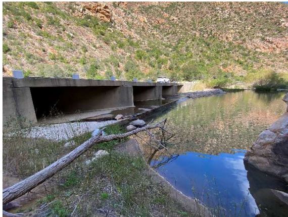
Repaired spalling and cracking observed downstream of Causeway No 4.
