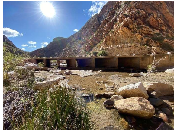
Repaired deck edge breaks and cement works evident downstream of causeway 18.
