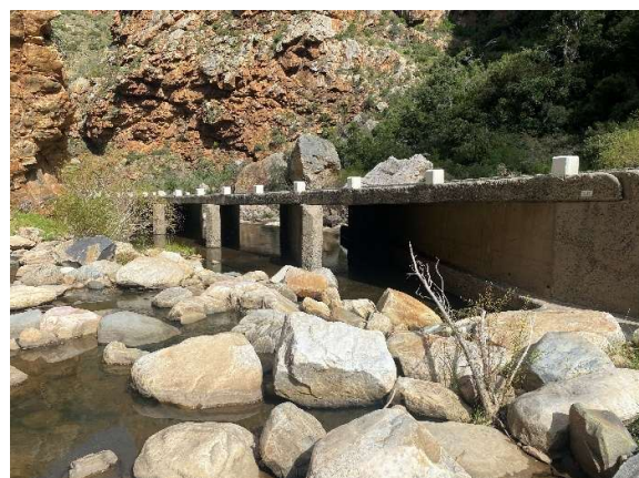
Repaired cell joint fillers, which has been dislodged during the recent floods.
