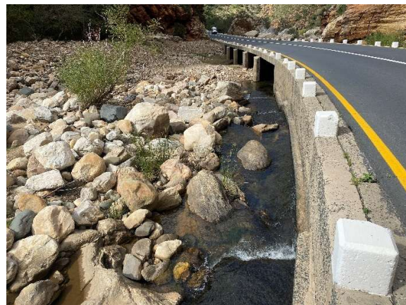
Upstream of causeway No 13 B2692A with no debris present and repair works evident.
