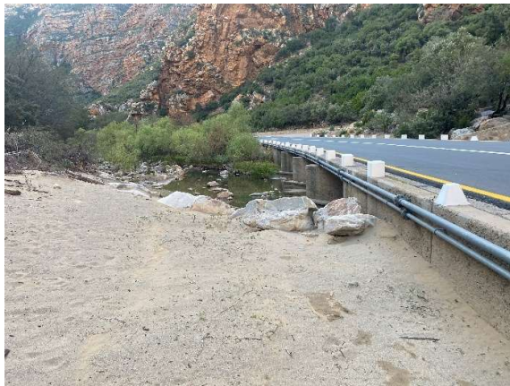
Potable water pipeline downstream of causeway 16 still in good condition. Some sedimentation present.
