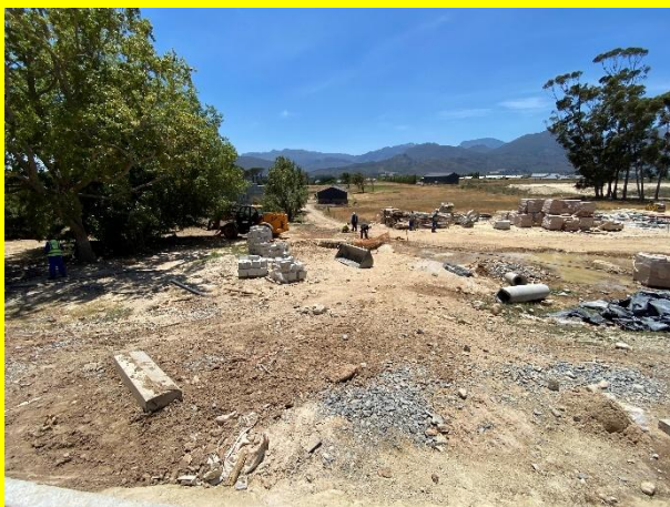
Construction material laydown area where the expansion is to occur. No buffer demarcation in place for wetland B
