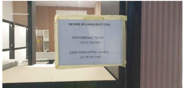
Emergency contact information available within the construction area of the mall.
