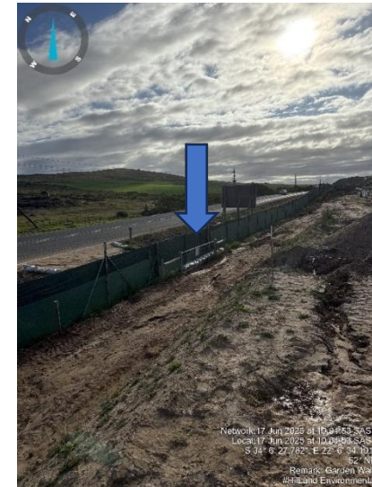
Additional sandbags were placed at the low point (old access point). Sandbags will be required here to protect the slope (soil erosion risk) until the retaining wall is completed.
