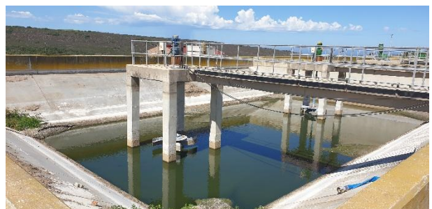
Existing biological reactor.
