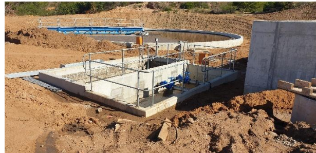
New Ras Pump Station in between new biological reactor and new clarifier.
