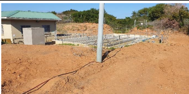
Fence wiring scattered around on site.
