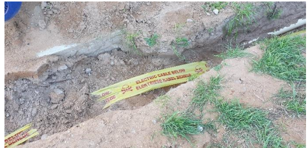
Notification of an electric cable running along the new mechanical dewatering facility.
