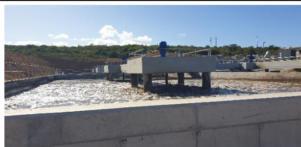
Newly installed and activated biological reactor.
