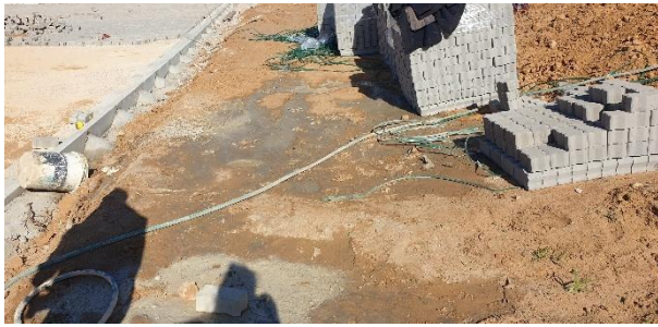
Ready mix cement residue adjacent to the ras pump station.
