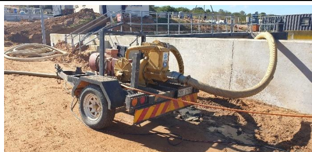
Dewatering centrifugal pump.
