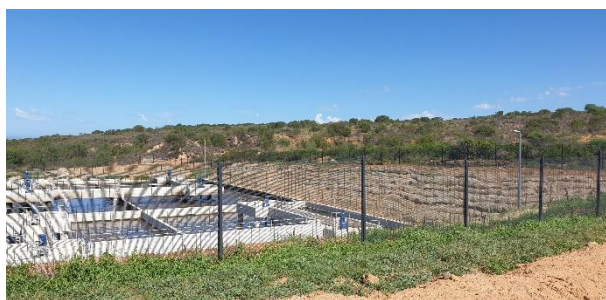
ClearVu Fence installed surrounding the WWTW plant.
