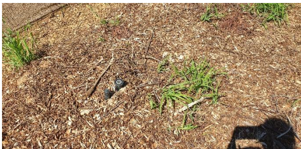
Irrigation system installed above the newly constructed clarifier.
