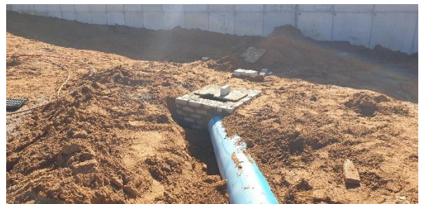
Stormwater system installed for redirecting surface runoff.
