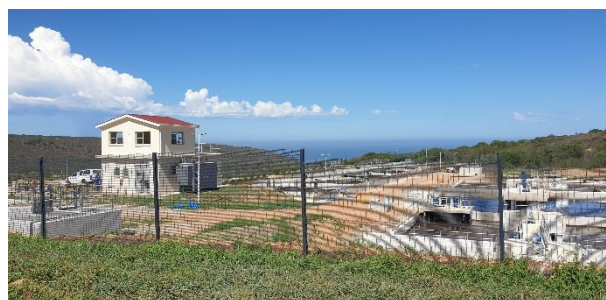
ClearVu Fence installed surrounding the WWTW plant.
