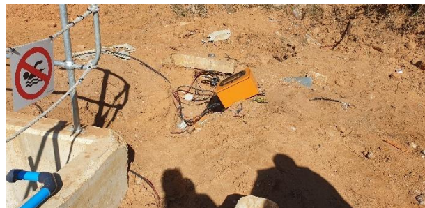
Electrical wiring is exposed adjacent to the existing chlorine channel.
