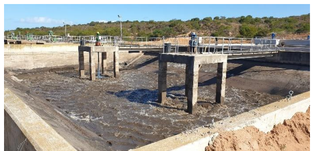
Existing biological reactor being pumped out.
