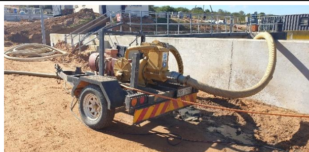
Dewatering centrifugal pump.
