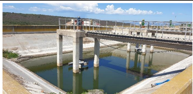
Existing biological reactor.
