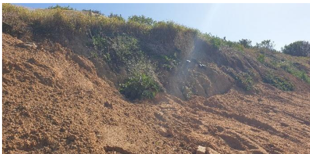
Historically, waste was dumped at the top of the slope on the northwestern edge of the new biological reactor.
