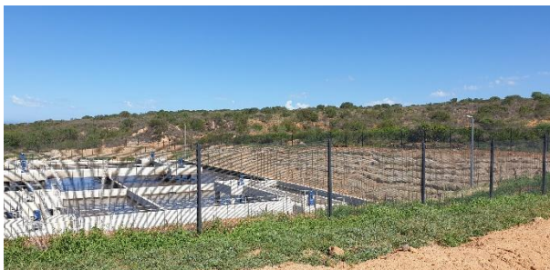
ClearVu Fence installed surrounding the WWTW plant.
