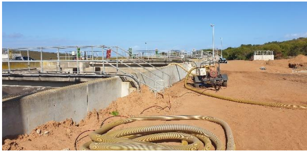
Existing biological reactor being pumped out.
