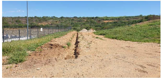
Stormwater/surface water diversion channel created at the entrance of the WWTW.
