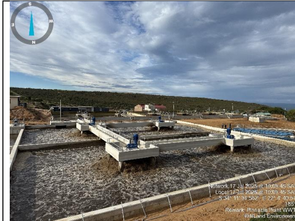
Reactors are being tested
