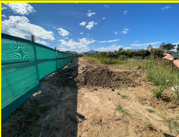
Buffer area along the wetland with material spoil which must be removed.
