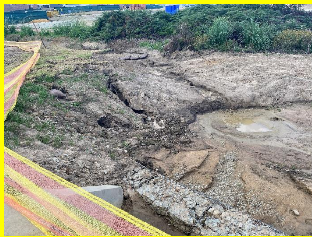
Stormwater outlets installed with energy dissipators (reno-mattress) in the wetland buffer area. Erosion should be monitored.
