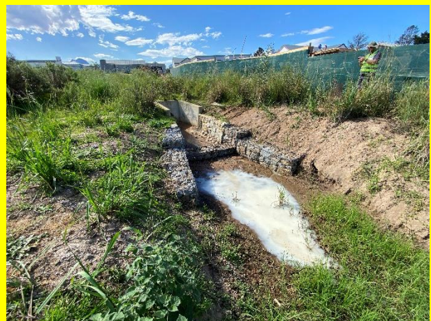
Paint was washed by contractors, resulting in paint residue entering the constructed stormwater outlet within the Phase 4B buffer area.
