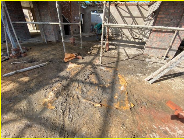
Construction of residences within Phase 3, cement batching on plastic sheeting is insufficient; proper mortarboards and catch pits are required.
