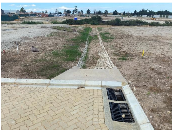
The sewer line and stormwater dissipator towards the north.
