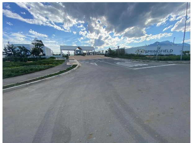
Condition of Providence Road at the Springfield Estate Entrance.
