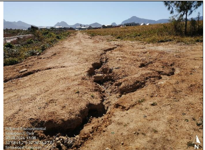
Phase 3 – sewer line must be rehabilitated and adequate erosion protection must be installed.
