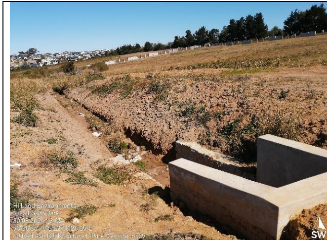
Stormwater outlets - sandbags (silt management) must be continuously maintained to reduce erosion and siltation downstream.
