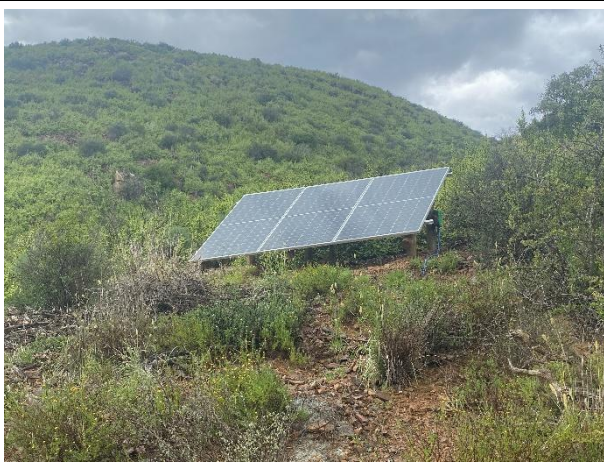
Solar panels at the entrance of the house.
