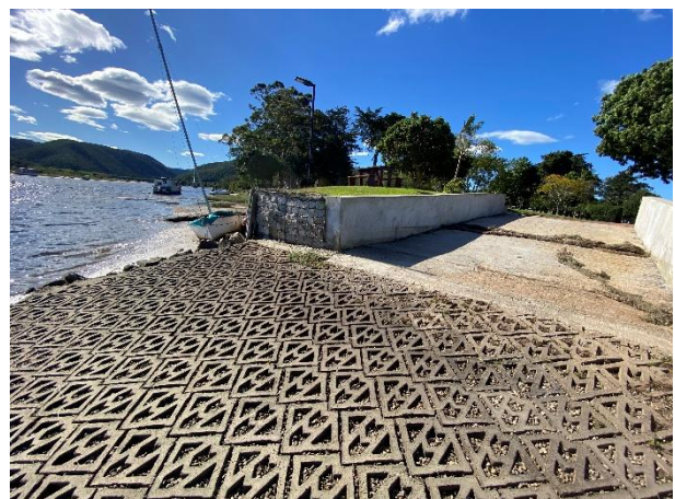
Condition of the slipway grassblocks.
