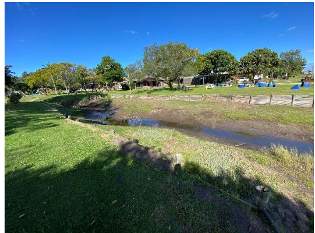
Condition of the stormwater channel outlet into the Keurboom River Estuary towards San Marino.
