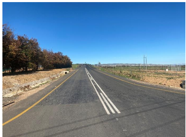
Condition of Protea Road, successfully resurfaced eastern end at the start of the contract.
