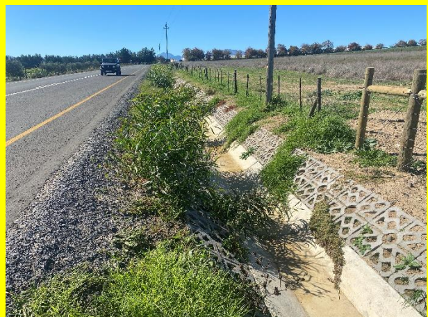
Golden Wreath Wattle observed establishing along the road reserve and stormwater channel.
