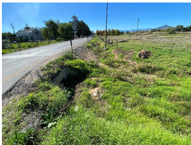
At the western end of Protea Road where stormwater culverts are installed adjacent to the road shoulder
