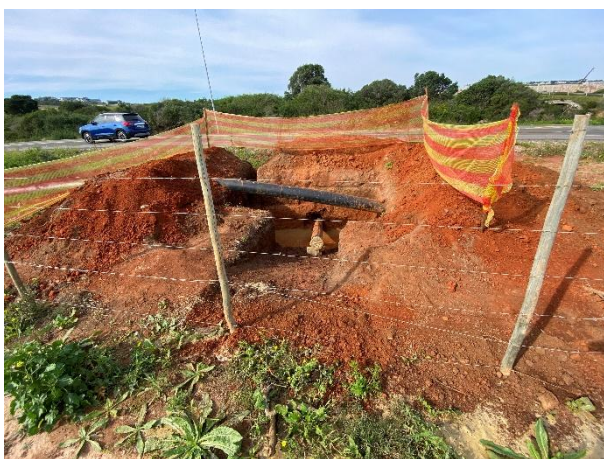
T-piece connection point adjacent to the R102.
