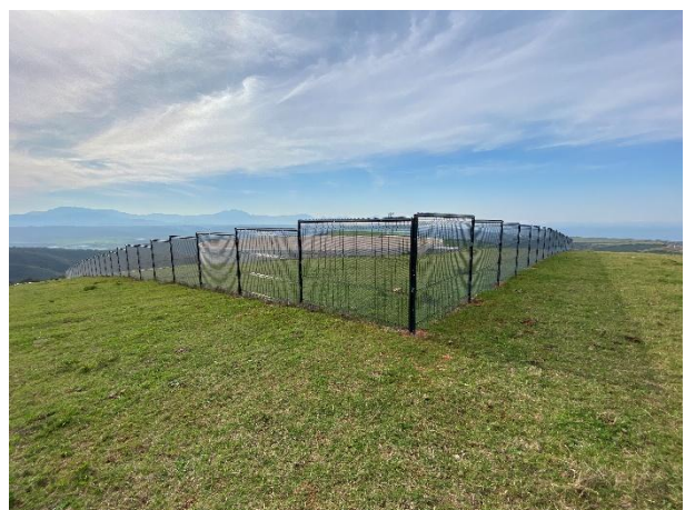
Existing 7 Ml reservoir fully fenced with ClearVu fencing.
