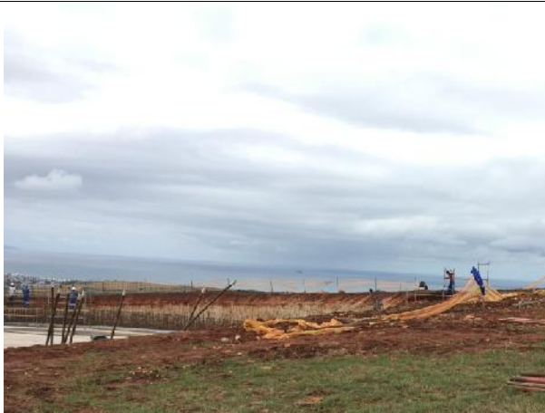
2021.03.17 – The No-Go demarcation around the excavation area is insufficient.
