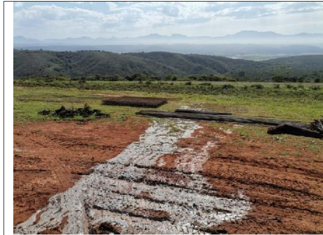
2021.04.21 – The cement run-off water MUST be prevented from flowing into the agricultural fields and natural vegetated area.
