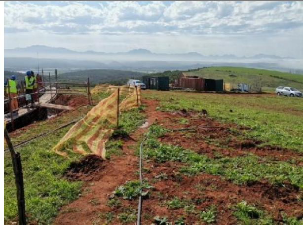
2021.04.21 – The orange netting is only installed on the southern edge.
