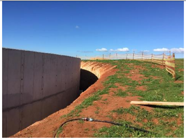
2021.05.12 – The orange netting is only installed on the southern edge; cattle can still enter the construction site where there is deep excavation.
