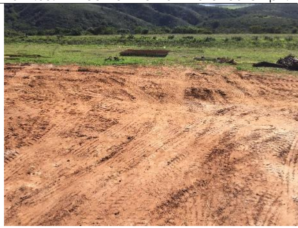
2021.05.12 – Cement run-off water was removed.
