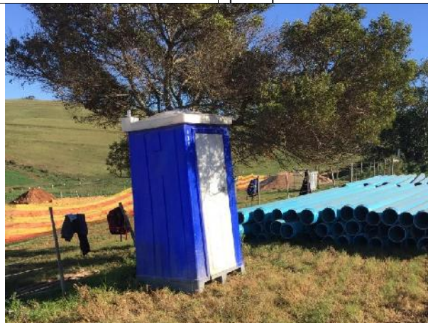
2021.06.17 – Ablution facilities available for pipeline staff.
