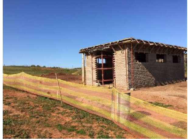
2021.08.23 – The No-Go demarcation around the pumpstation.
