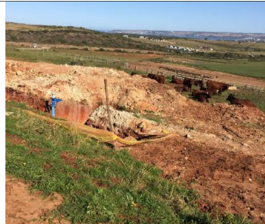
2021.08.23 – The contractor is reminded that orange netting must be used to demarcate deep trenches, especially in the camps where the cattle are grazing.
