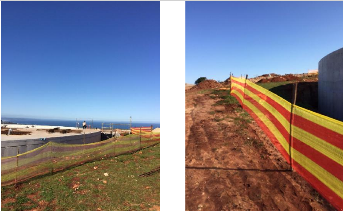
2021.08.23 – The demarcation is in place. The contractor must ensure that it is maintained and fully upright before leaving the site each day.
