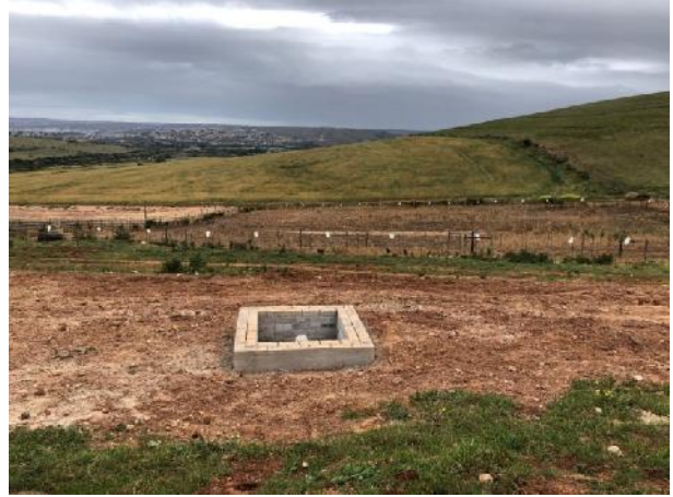
2021.09.27 – Demarcation of deep trenches must be in place – manholes have been constructed and must be demarcated until they are fully covered to prevent farm animals from accidentally injuring themselves.
