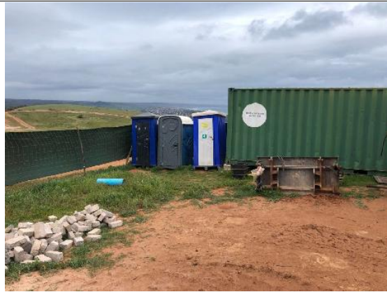
2021.09.27 – Ablution facilities is available for all staff on site.
