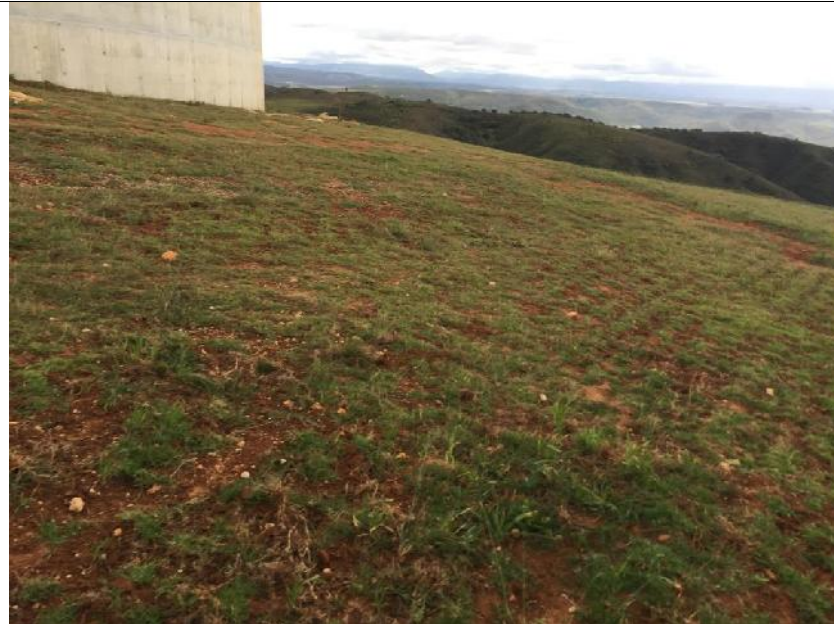
Compacted soil was loosened, and grass is growing
